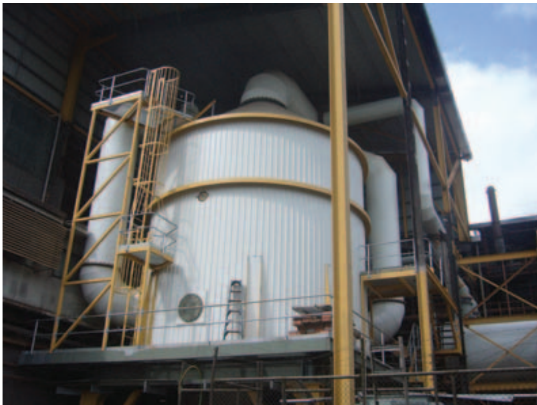
Evaporator, South Johnstone mill (North Queensland, Australia)
